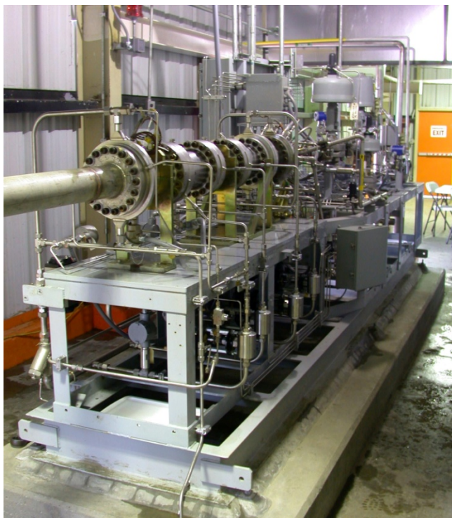
Clean Energy Systems' Oxy-Combustion 5MWe Gas Generator
